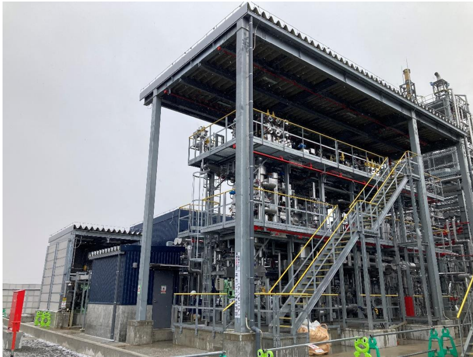
Image: Small ammonia synthesis facilities installed at INPEX as Tsubame BHB's first commercial facilities
